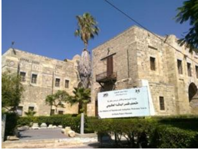
Rehabilitation of Basha Palace and converting it into a museum Source : The Researcher
