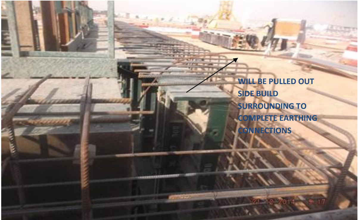
4- INCREASE THE LENGTH OF EARTING TERMINAL AROUND 3M TO FUTURE CONNECYION AFTER CASTING.
