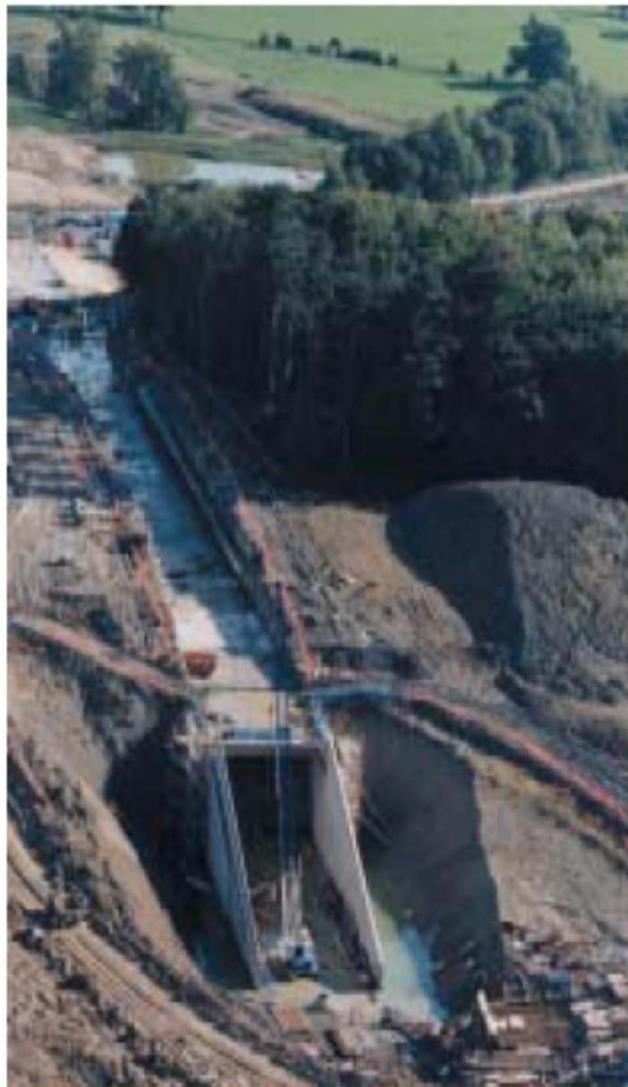
8. Boxley Tunnel, which passes through an area of ancient woodland that had to be conserved.
