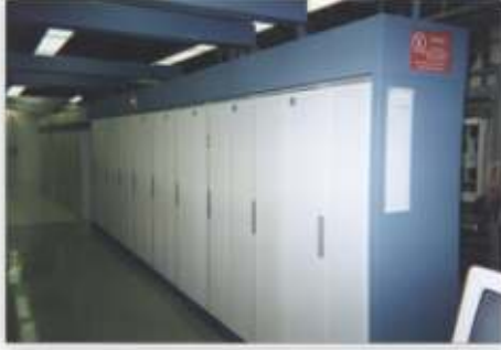
Large Telephone Switches
