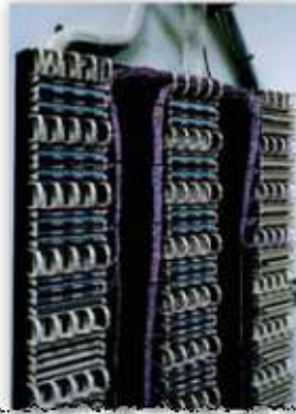
Wiring Closet Infrastructure
