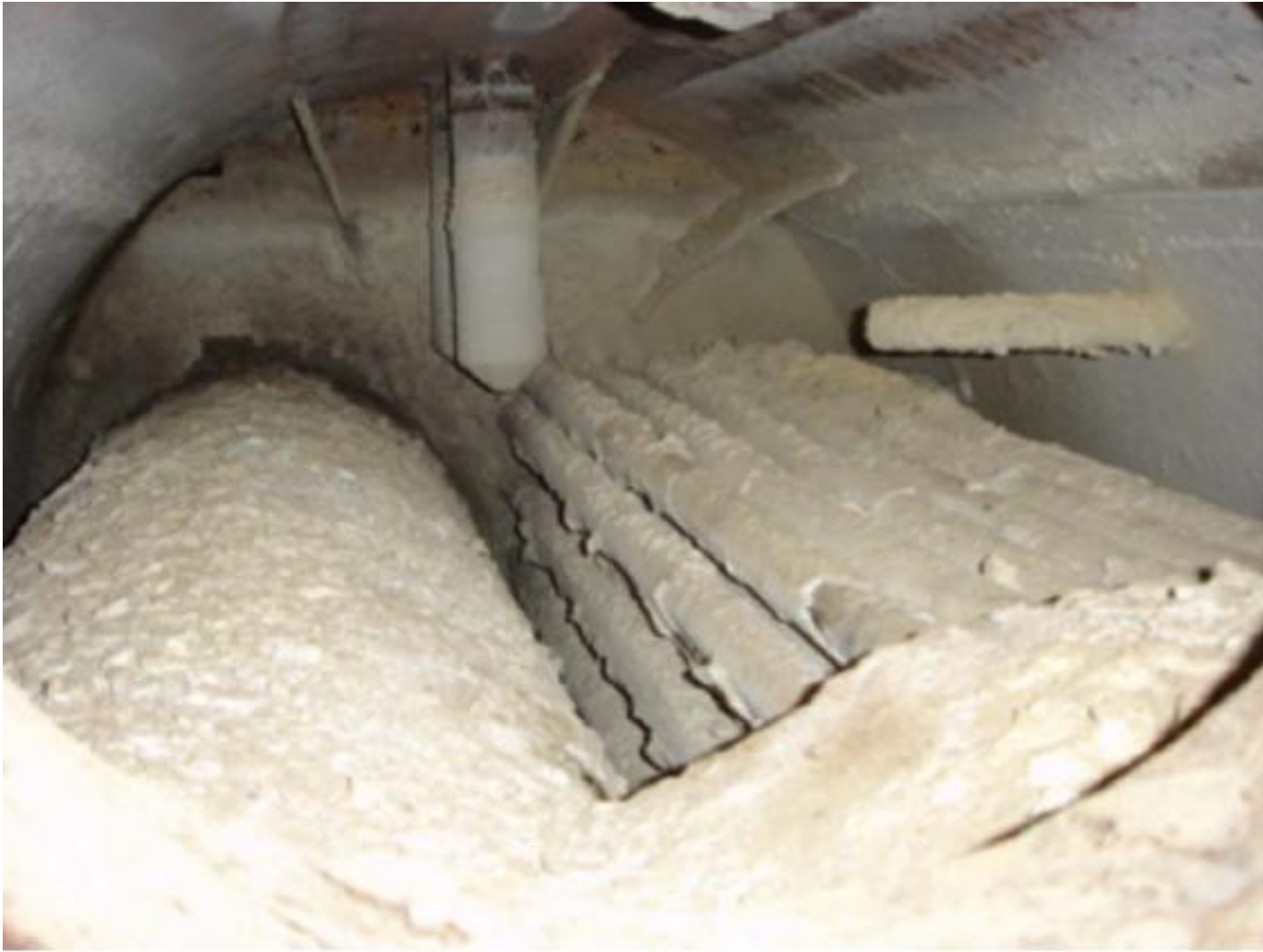
Figure 2: Consequences of inadequate hardness monitoring
