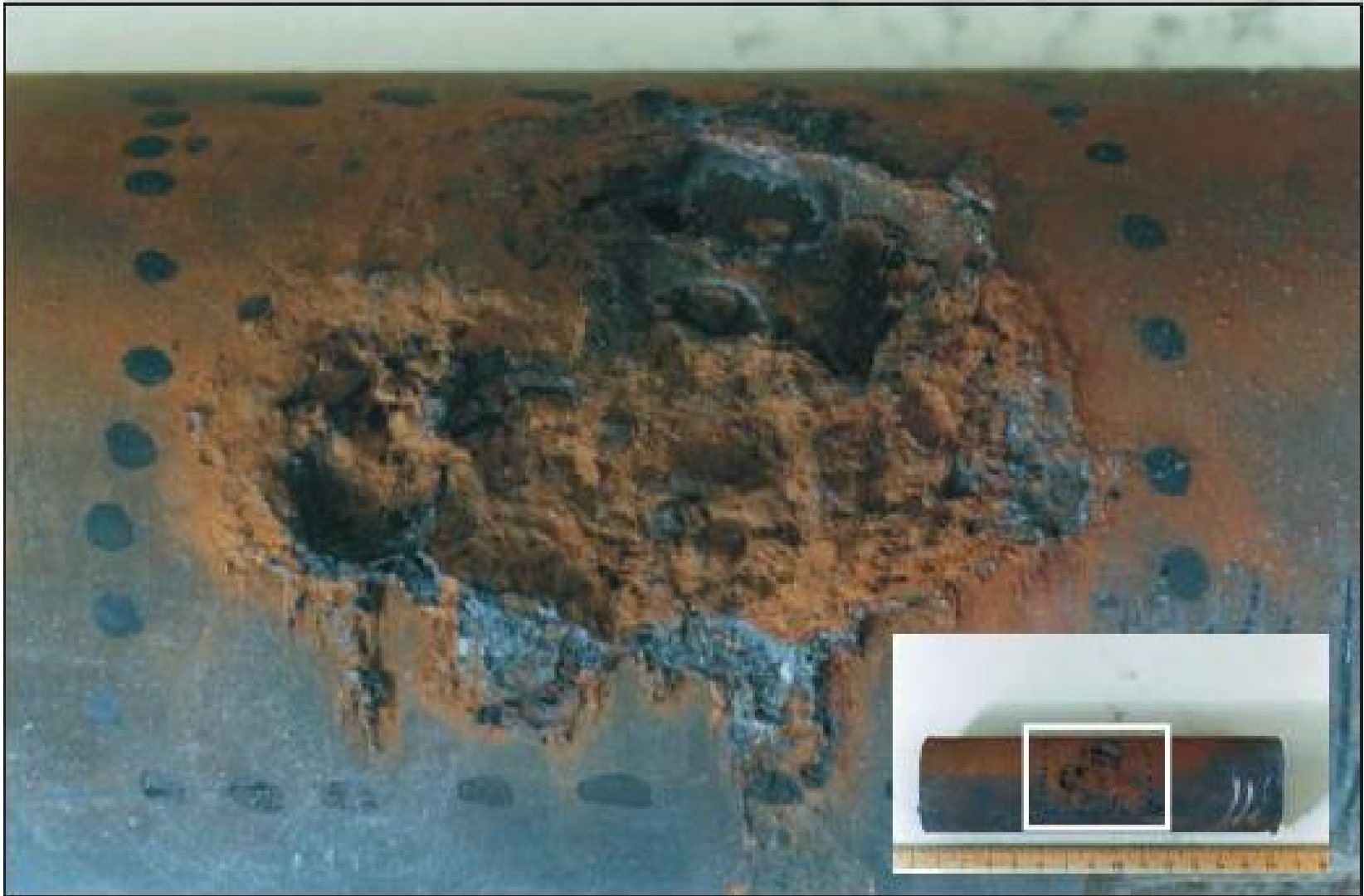
Oxygen attack on a cut-out smoke tube
